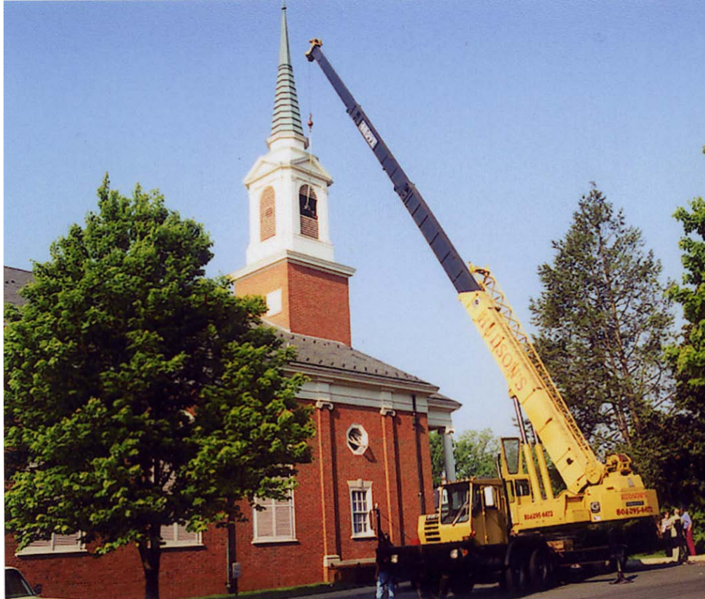
A crane was used to hoist the large 960 pound bell toward the steeple.
